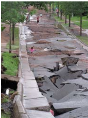
Changing weather patterns put key infrastructure at risk
