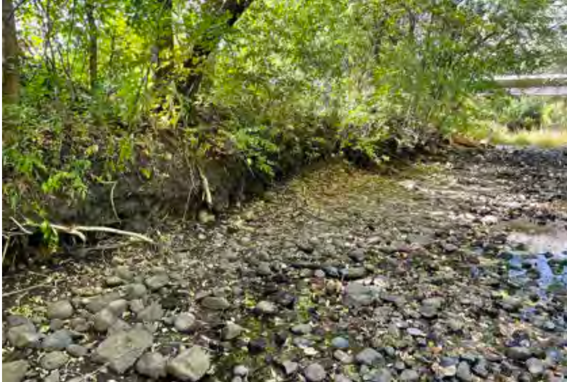
Figure 4: Bank erosion downstream of Cedar Lake Trail crossing.
