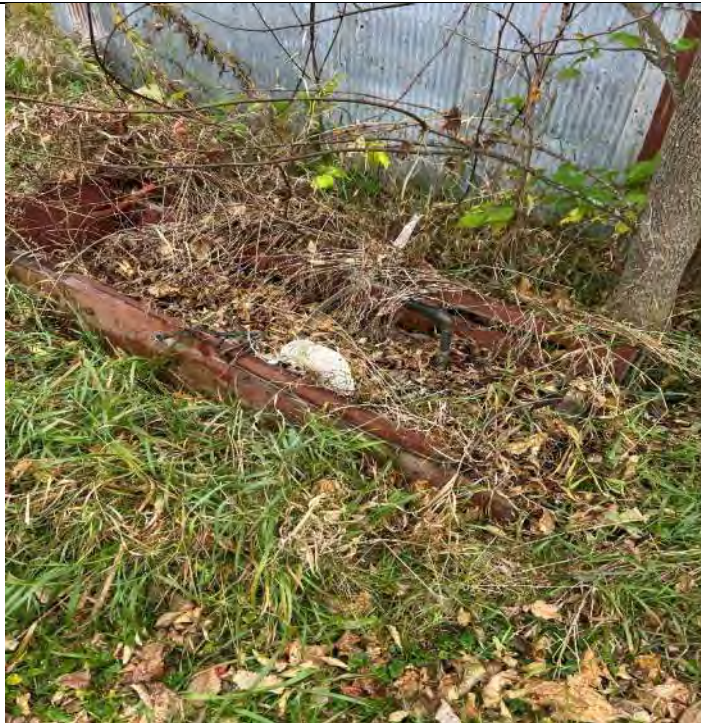
Photo #9 Typical of former wooded stand with pump and surface piping north of centrally located shed.
