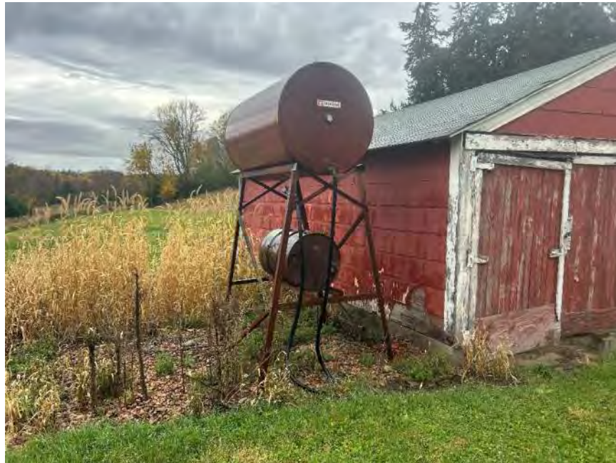
Photo #4 View of ASTs on metal stand south of shed.
