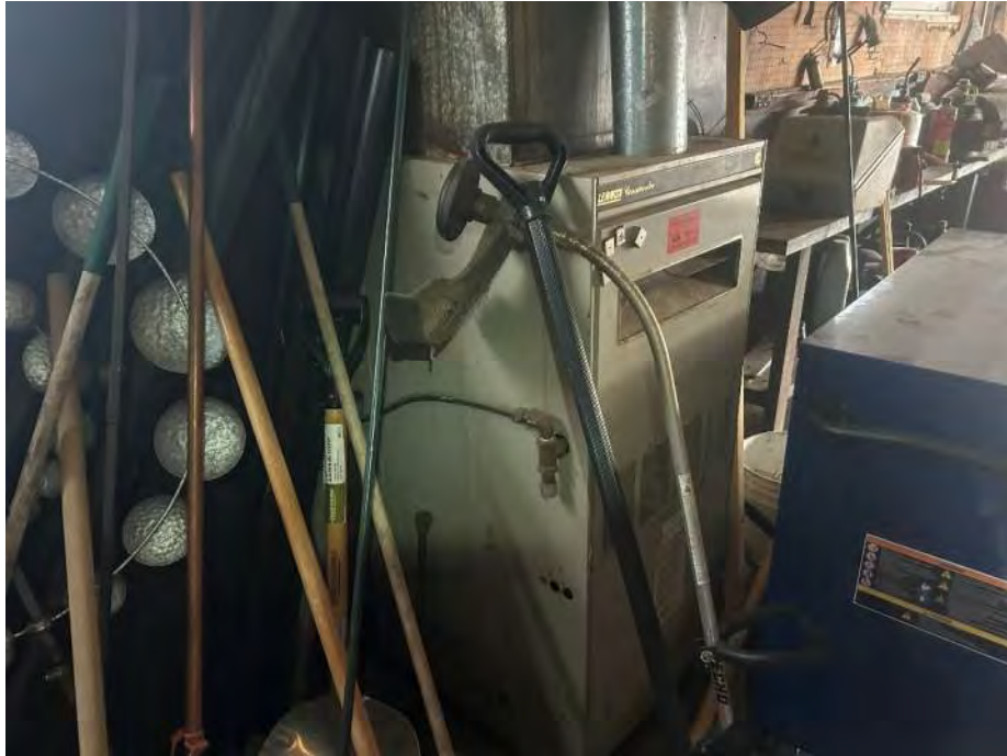
Photo #13 View of furnace in garage, east of residence.
