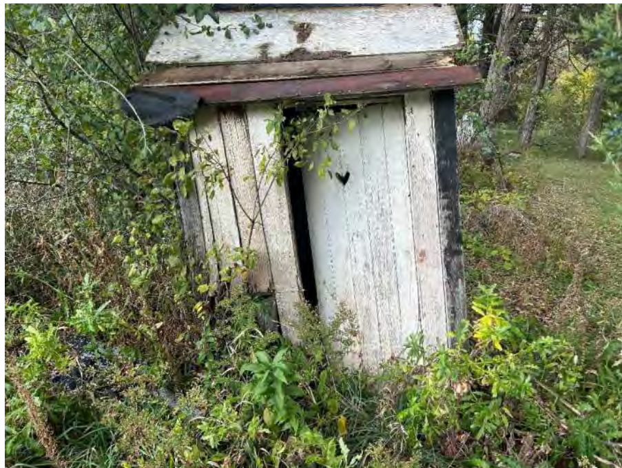
Photo #18 View of dilapidated outhouse west of residence.
