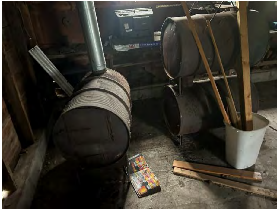
Photo #15 View of wood burning stoves in one of wood sided sheds.
