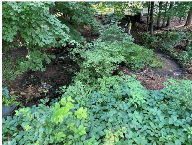
Existing depressed area south of Morningside Rd providing pretreatment. Photos taken in July 2023.
