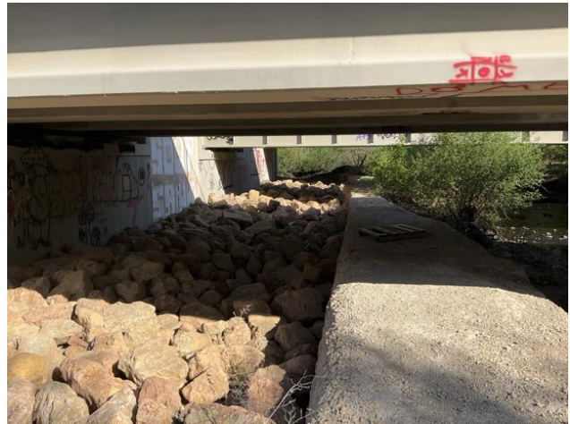
Photo 20. View of upland point PP06 under the trail and railroad bridges over Minnehaha Creek. Upland riprap and concrete wall present on west side of creek under bridges. Photo taken facing north.
