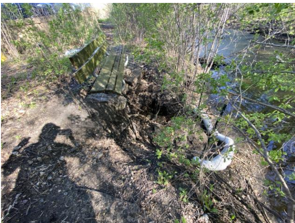
Photo 17. View from PP04. Note some erosion into the bank from the creek at the foot of the bench. Photo taken facing west.
