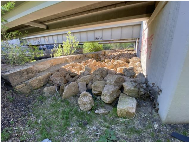
Photo 21. View from upland point PP07 of riprap under the bridges. Photo taken facing south.
