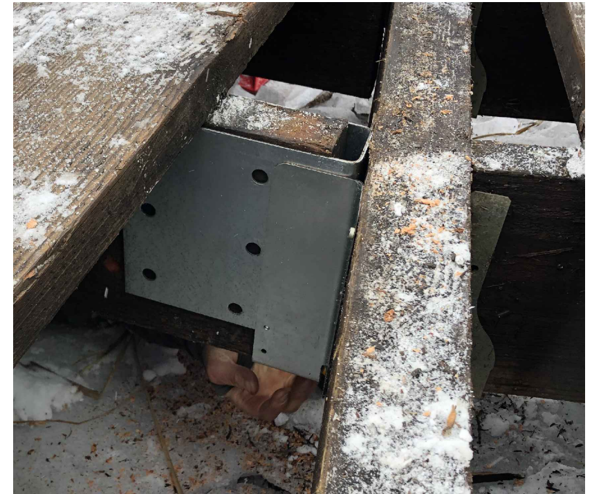
GAPS GREATER THAN 5/8" UP TO 1 1/4" REPAIR IMAGE OF JOIST EXTENSION BRACKET INSTALLATION FIELD TEST (CUSTOM MITEK PRODUCT EC-SB23-0509A)
