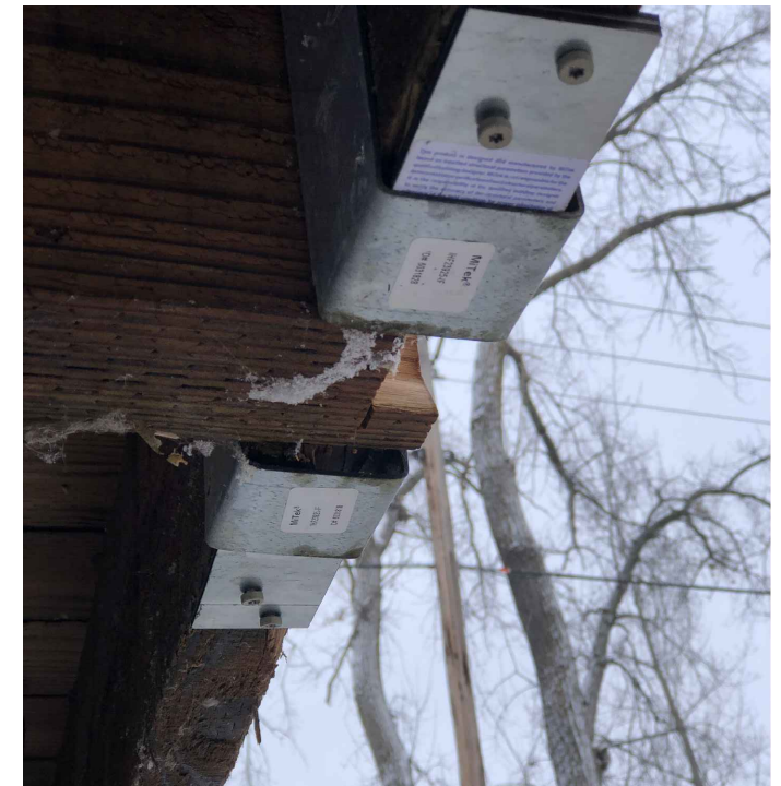
RESTRAINED BEARING PLATES REPAIR IMAGE OF RESTRAINED BEARING PLATES FIELD TEST (CUSTOM MITEK PRODUCT EC-TG23-1023)
