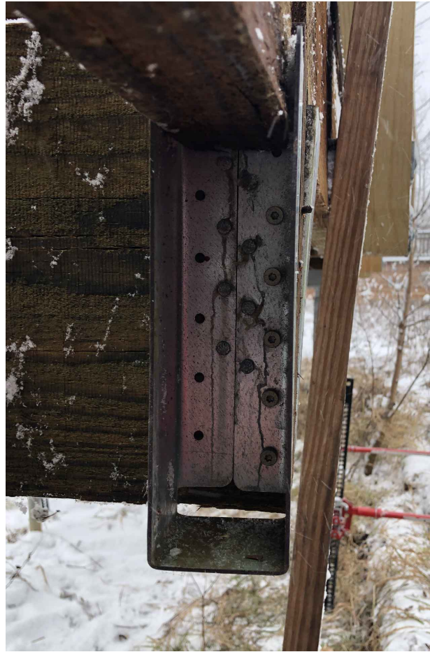
MAXIMUM FASTENER SCHEDULE REPAIR IMAGE OF SUPPLEMENTAL FASTENERS FIELD TEST (CUSTOM MITEK PRODUCT LL930 SCREWS)
