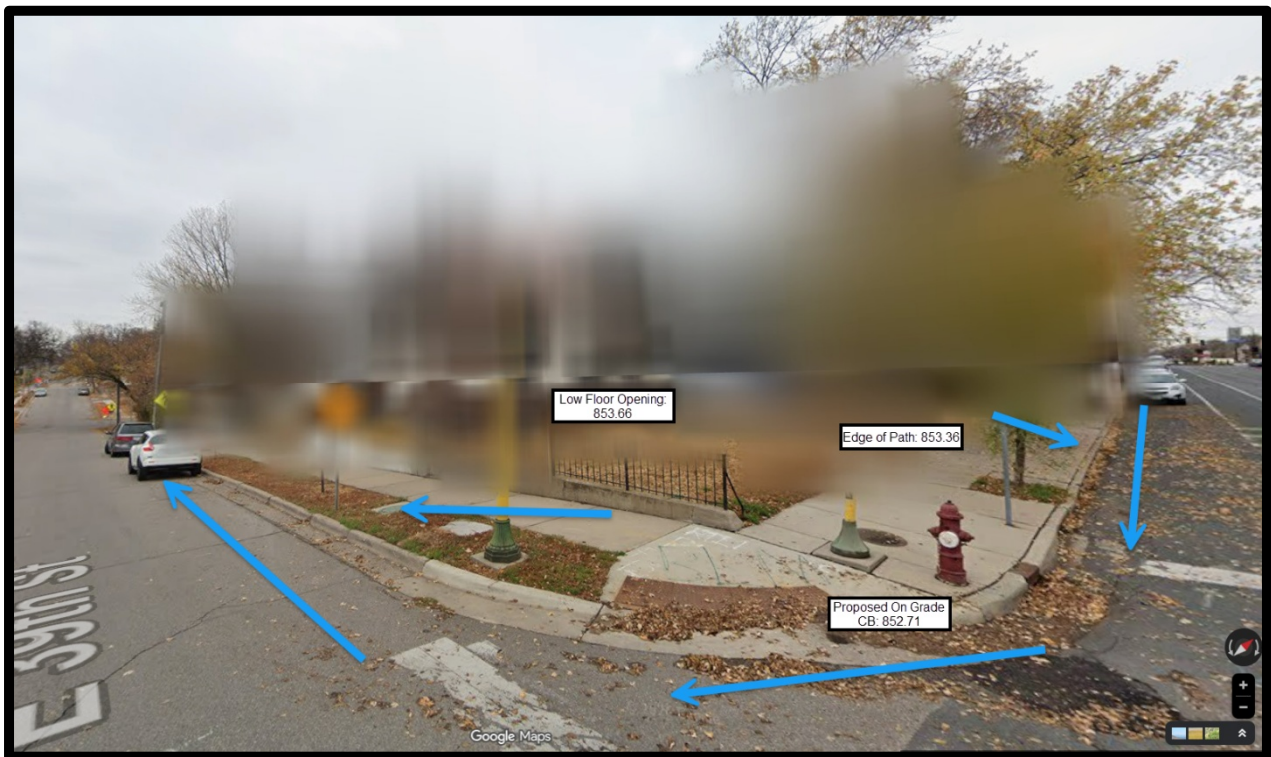
Chicago Ave (West Side) Residence Low Opening & Runoff Pattern
