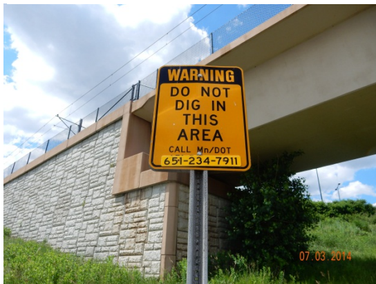
Figure 8 - GLS Warning Sign
