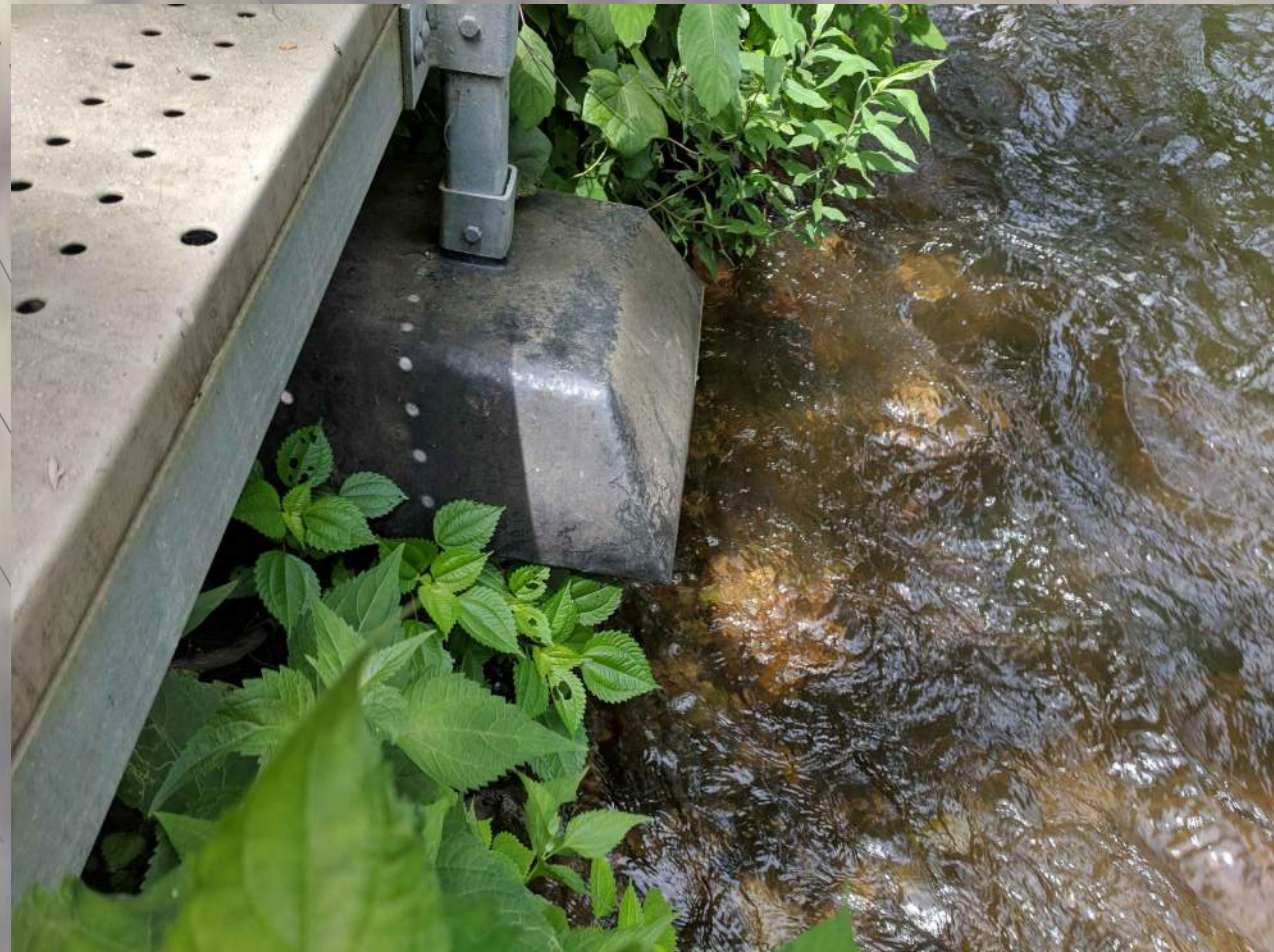
PHOTO - PROJECT 5 LOOKING NORTHWEST AT UNDERMINED FOOTING
