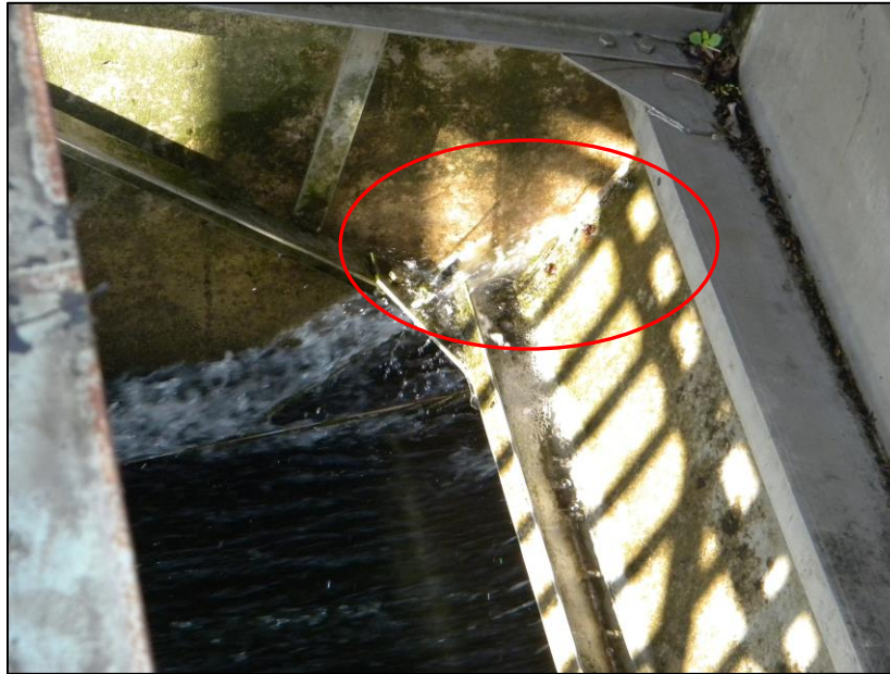
Westerly Gate Seal Leakage – May 12, 2016
