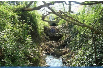
Library Parking Lot Outfall—Before
