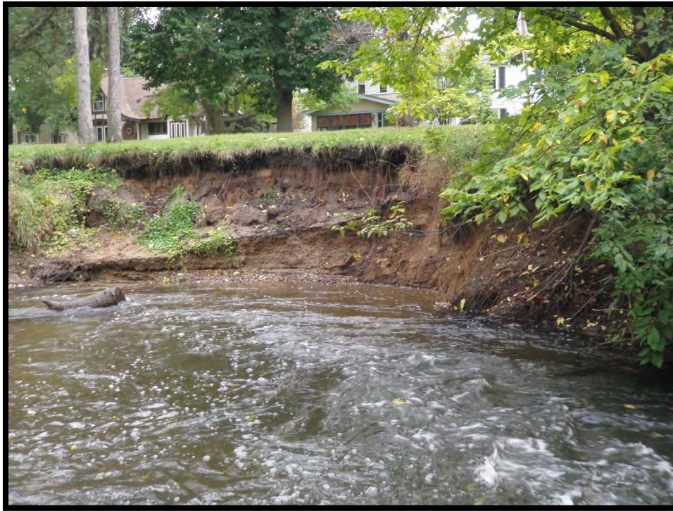
Erosion along Minnehaha Creek near Portland Ave S in Minneapolis
