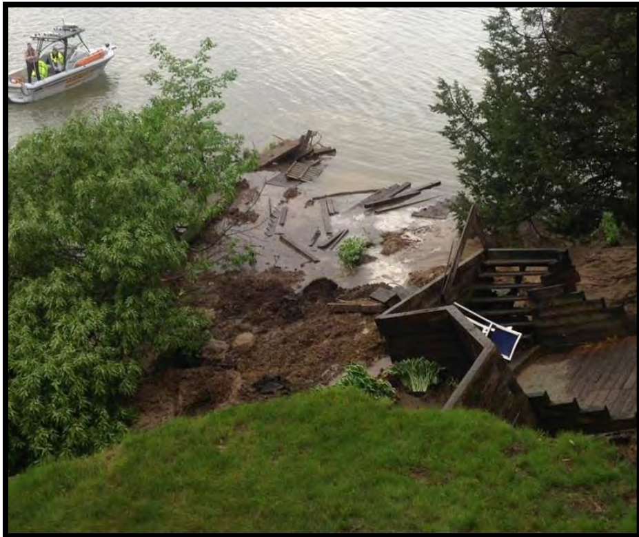
Slope Failure on Lake Minnetonka near Woodside Lane in Shorewood
