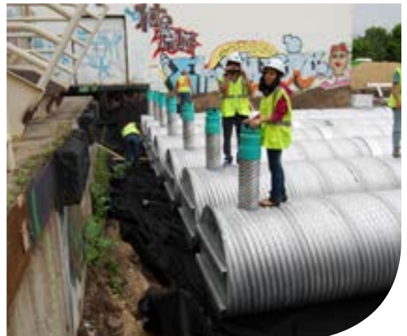
Underground stormwater treatment in Minneapolis
