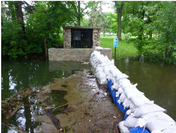
Figure 1. Sand bags were placed on top of the dam to hold back water from entering Lake Nokomis.
