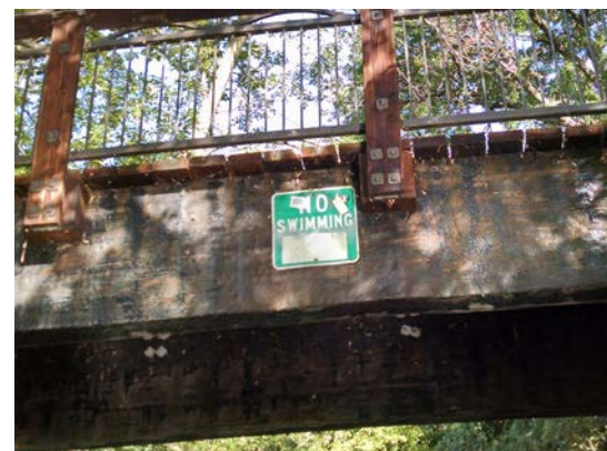
69 Minnehaha Creek Hazard - No Swimming, 36th Ave
