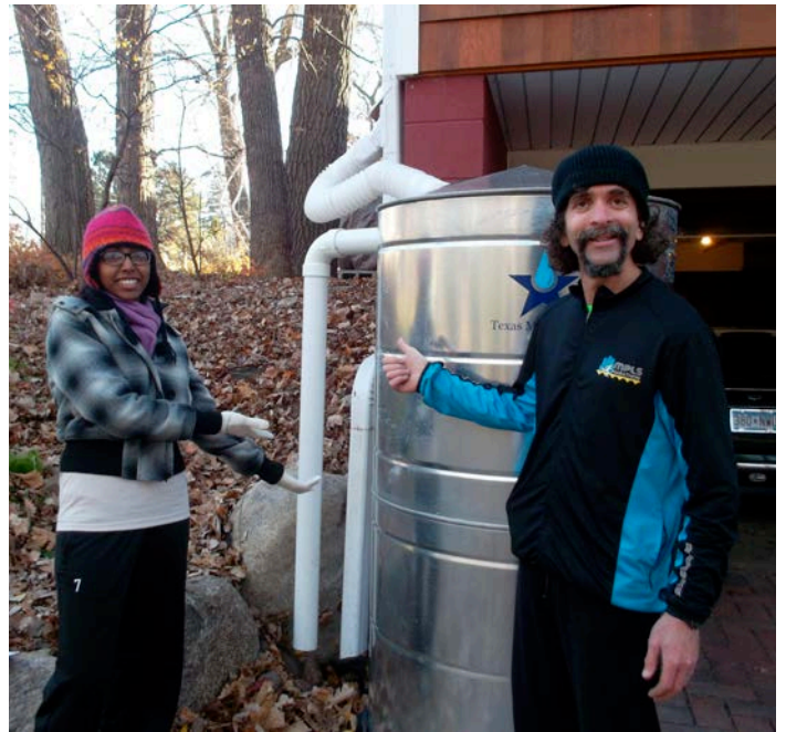
Stewards standing in front of their recently-installed "cistern," which catches rain to re-use instead of letting it flow into the street
