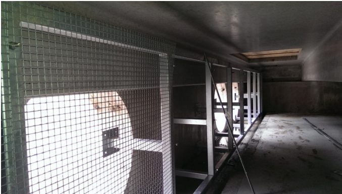
Structural framing and steel backer screen construction for curtain wall pre-treatment system. When complete, a sacrificial filter fabric will be mounted against the backer screen to filter fine particles from entering the three 48-inch openings to the infiltration system. A large vault opening indicated in upper right (background) of photo allows maintenance access for periodic removal and replacement of fabric.
