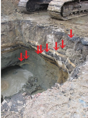
Excavation to fix exterior watermain break at existing mall. At least eight distinct repaving layers apparent extending about 6-feet below grade.
