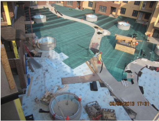
Under the charm – construction of waterproofing and drainage systems prior to adding soil media and plants on the green roof of the Folkestone Terrace West (fka, Superior Block). Photo courtesy of Adolfson & Peterson Construction.
