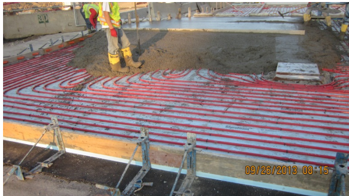
Concrete pour over hydronic snow-melt tubing around stormwater inlet grate at street intersection of The Promenade of Wayzata.
