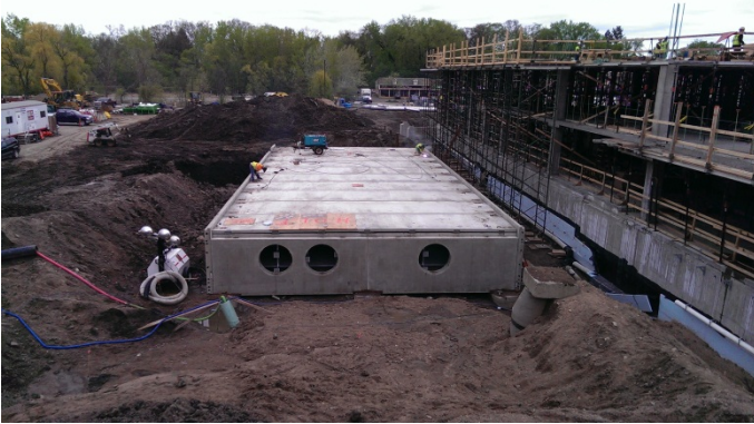
Looking south at Engel Street detention vault during construction. Three large openings are for connecting 48-inch perforated pipe network of adjacent infiltration basin.
