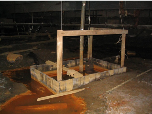
Makeshift sump pump to manage constant water in “crawl space” below existing mall.
