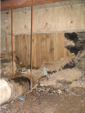
Roof pipe (white) connected to exterior storm sewer (black) – a flexible coupling between the two pipes is under stress from exterior settlement at the existing mall.
