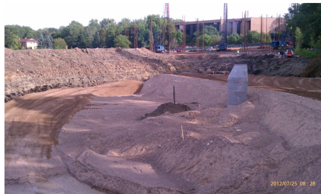
Imported clean sand fill in excavation for Engel Street infiltration basin (foreground). Steel pipe pile driving for Phase 1 building (background).
