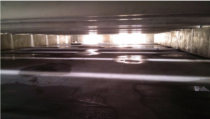
Looking north inside Engel Street detention vault during construction. Large sun-filled openings are for eventual connection with 48-inch perforated pipe network of adjacent infiltration basin.
