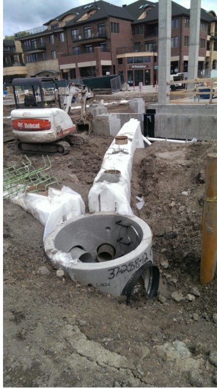
Storm sewer at The Promenade of Wayzata uses lightweight insulation "backfilled over pipes with poly sheeting "slip sheets" on sidewalls. Sonotubes centered over hanger connectors to be filled with reinforced concrete during subsequent post-tension slab pour.
