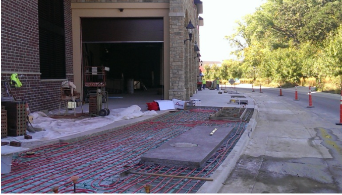
Hydronic snow-melt piping in walk by loading dock exit along Superior Boulevard at The Promenade of Wayzata.
