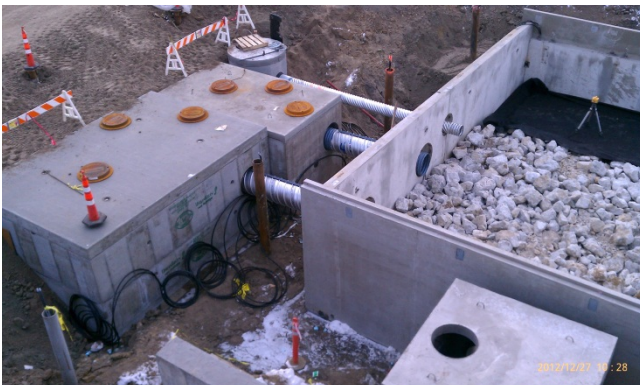
Large oil-grit swirl chambers over-pretreat boulevard runoff before discharging into the Mill Street filtration basin.
