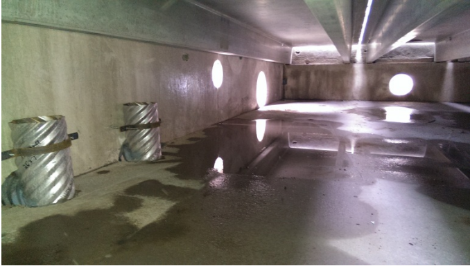
Two riser pipes for overflow of surficial portion of very infrequent storms rigidly connected to detention vault wall at south end of precast stormwater detention vault of Engel Street infiltration system (foreground). Riser rims set at 2.4-inch storm level, resulting in infiltration for 99% of annual rainfall for 5-acres of mostly impervious surfaces.
