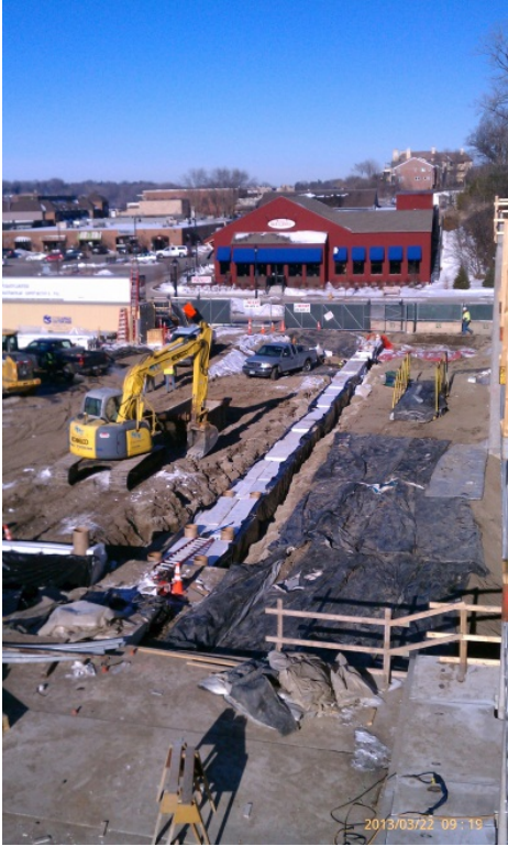
Storm sewer extending from Mill Street filtration basin. Lightweight insulation "backfilled" over pipes with poly sheeting "slip sheets" on sidewalls. Sonotubes centered over hanger connectors to be filled with reinforced concrete during subsequent post-tension slab pour at The Promenade of Wayzata.
