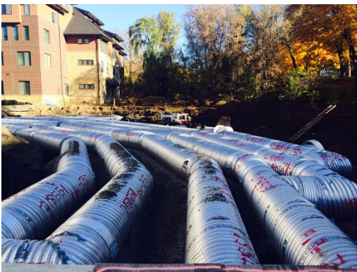
Perforated 48" corrugated metal pipe infiltration pipe installation at Engel Street infiltration basin. No alternative support for pipes is required since the soils on which the pipes bear are corrected inside the SCISZ. {SEE DRONE FLY-OVER OF THIS SYSTEM IN MID CONSTRUCTION @ www.youtube.com/watch?v=1iz_thP_1c&feature=youtu.be } Photo courtesy of Contech.
