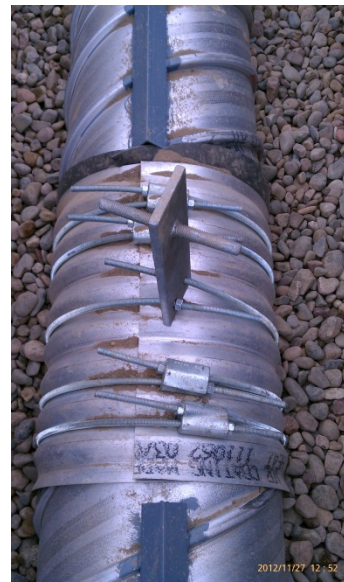
Hanger connector for storm sewer at The Promenade of Wayzata.
