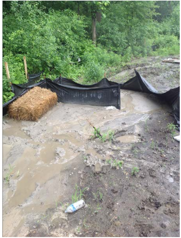
Failing erosion control documented 6/18/18
