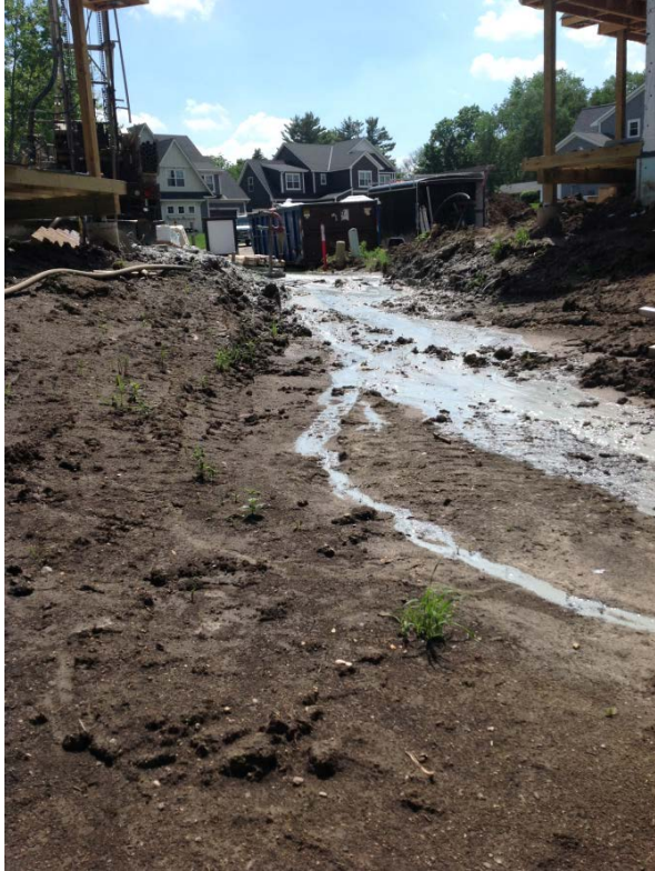
Illicit Discharge flowing through site 5/31/18
