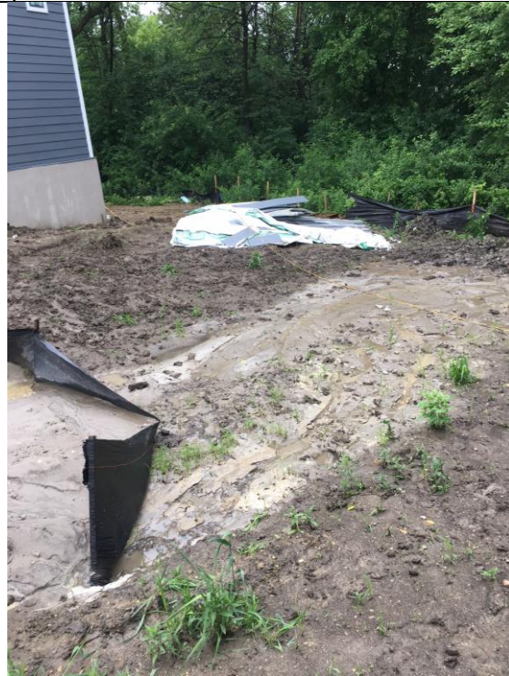
6/19/18: Silt fence overloaded by bentonite material
