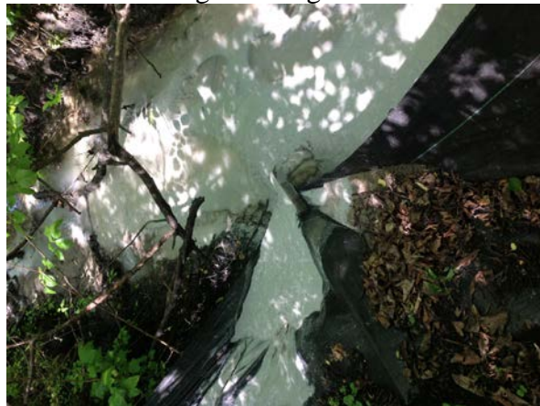
Failing erosion control, Illicit Discharge entering adjacent stream 5/31
