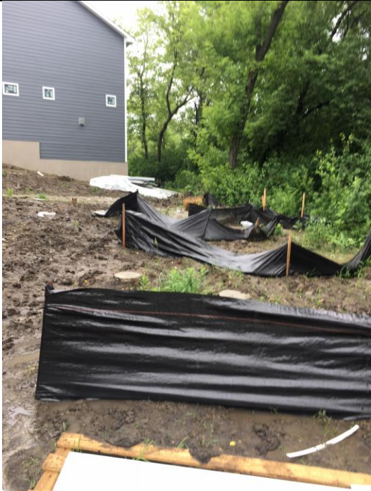
6/19/18: Redundant silt fence in development in need of maintenance
