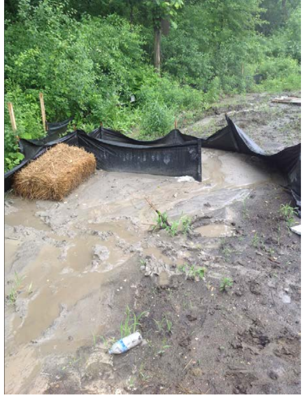
Failing erosion control documented 6/18/18
