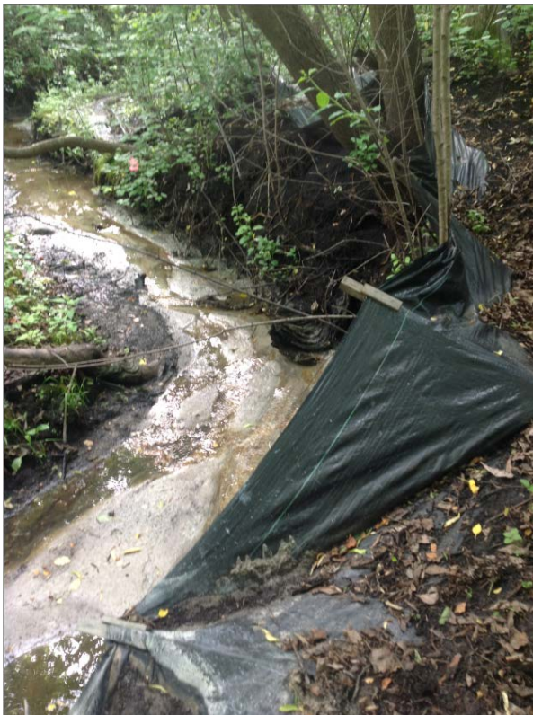
Illicit Discharge and failing erosion control documented on 6/8/18
