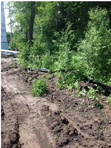
Failing silt fence around perimeter
