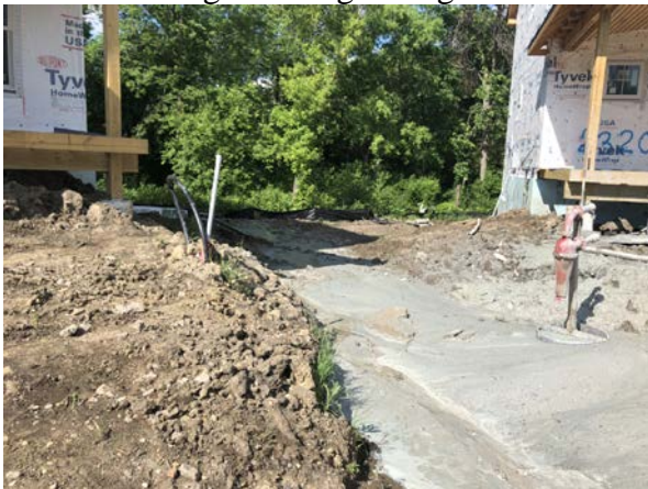
Illicit Discharge flowing through site 5/31/18
