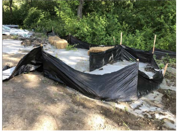
Failing erosion control documented 6/15/18
