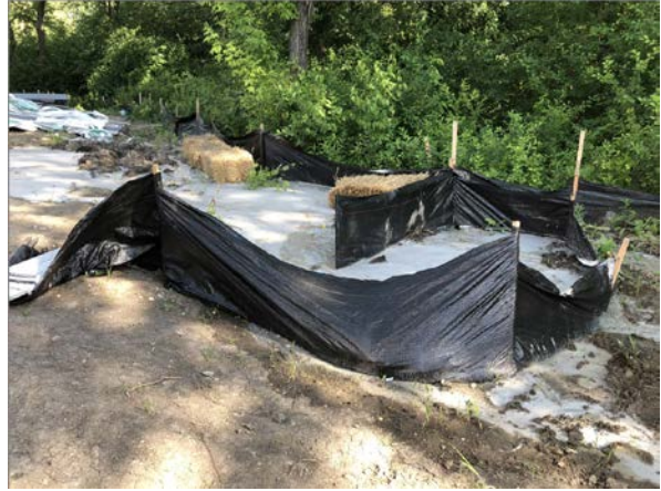
Failing erosion control documented 6/15/18
