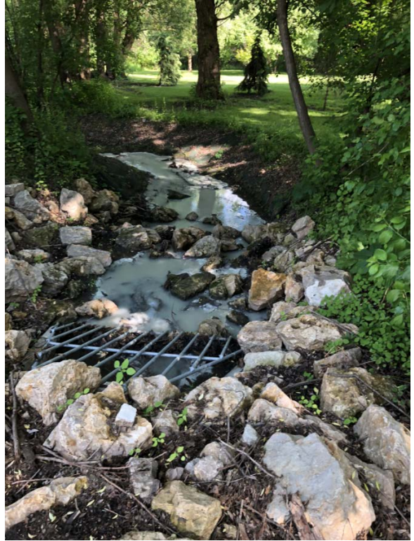
Illicit Discharge within stream at Watertown Road intersection 5/31/18
