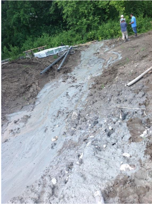
Illicit discharge draining towards wetland and stream
