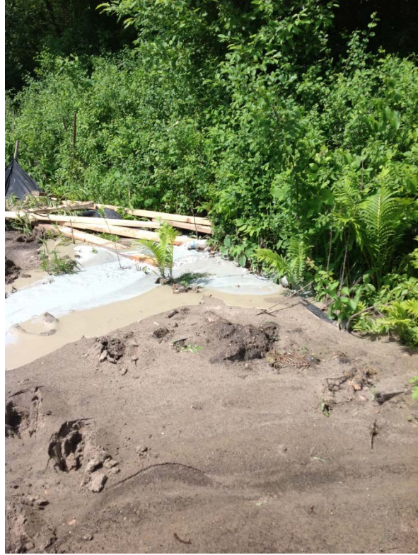
Illicit Discharge flowing off-site 5/31/18
