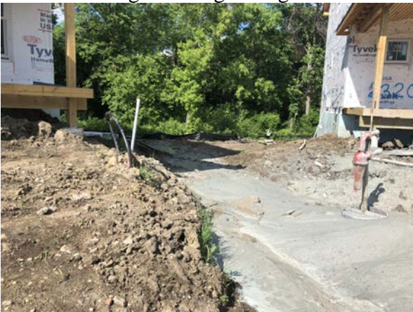
Illicit Discharge flowing through site 5/31/18
